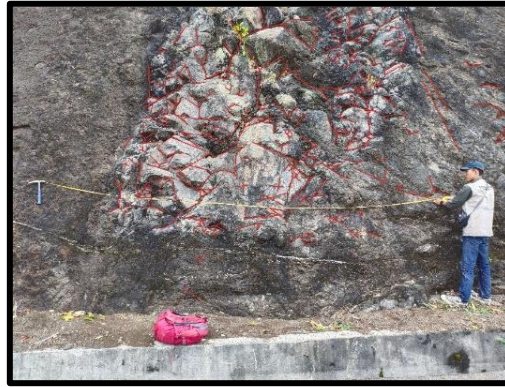
Fig. 6. Appearance of scouring bridle structure on the slope of andesite lithology at observation station 1.
